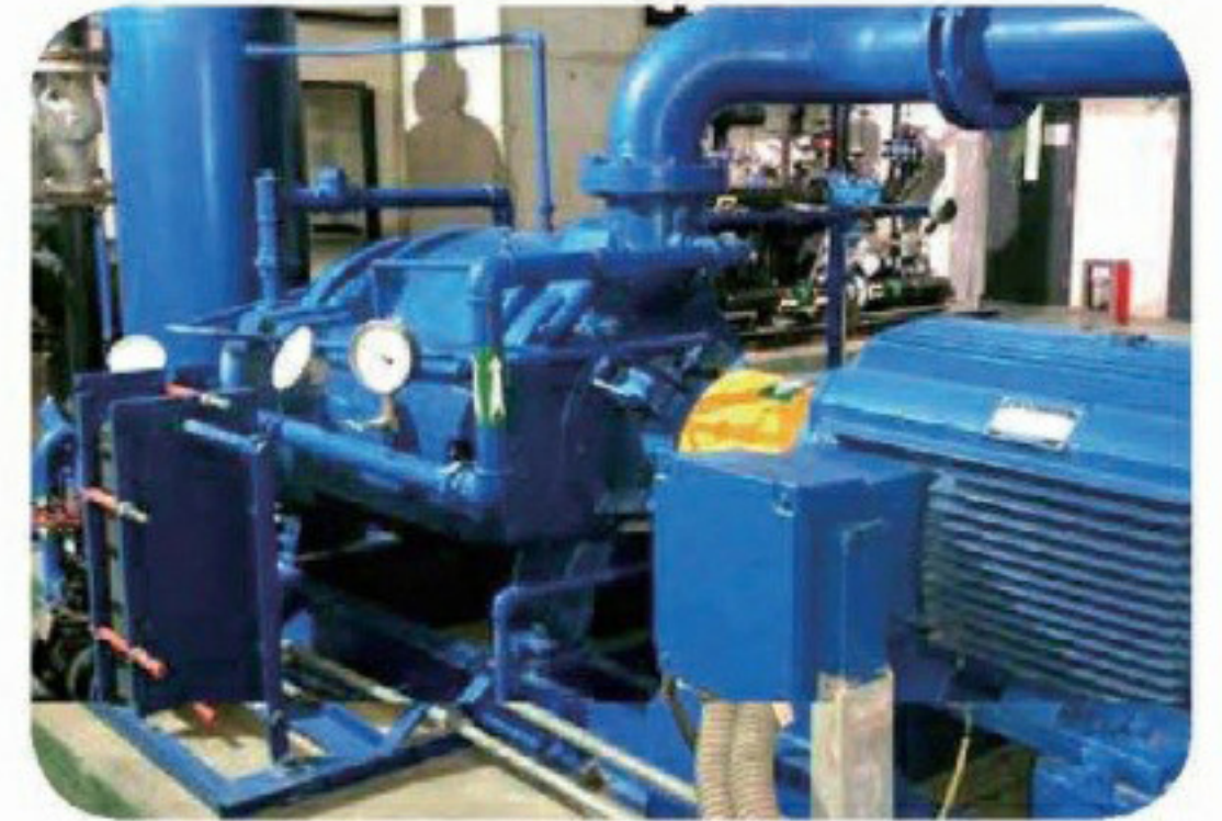
凝汽器抽真空 / Condenser Vacuum System
