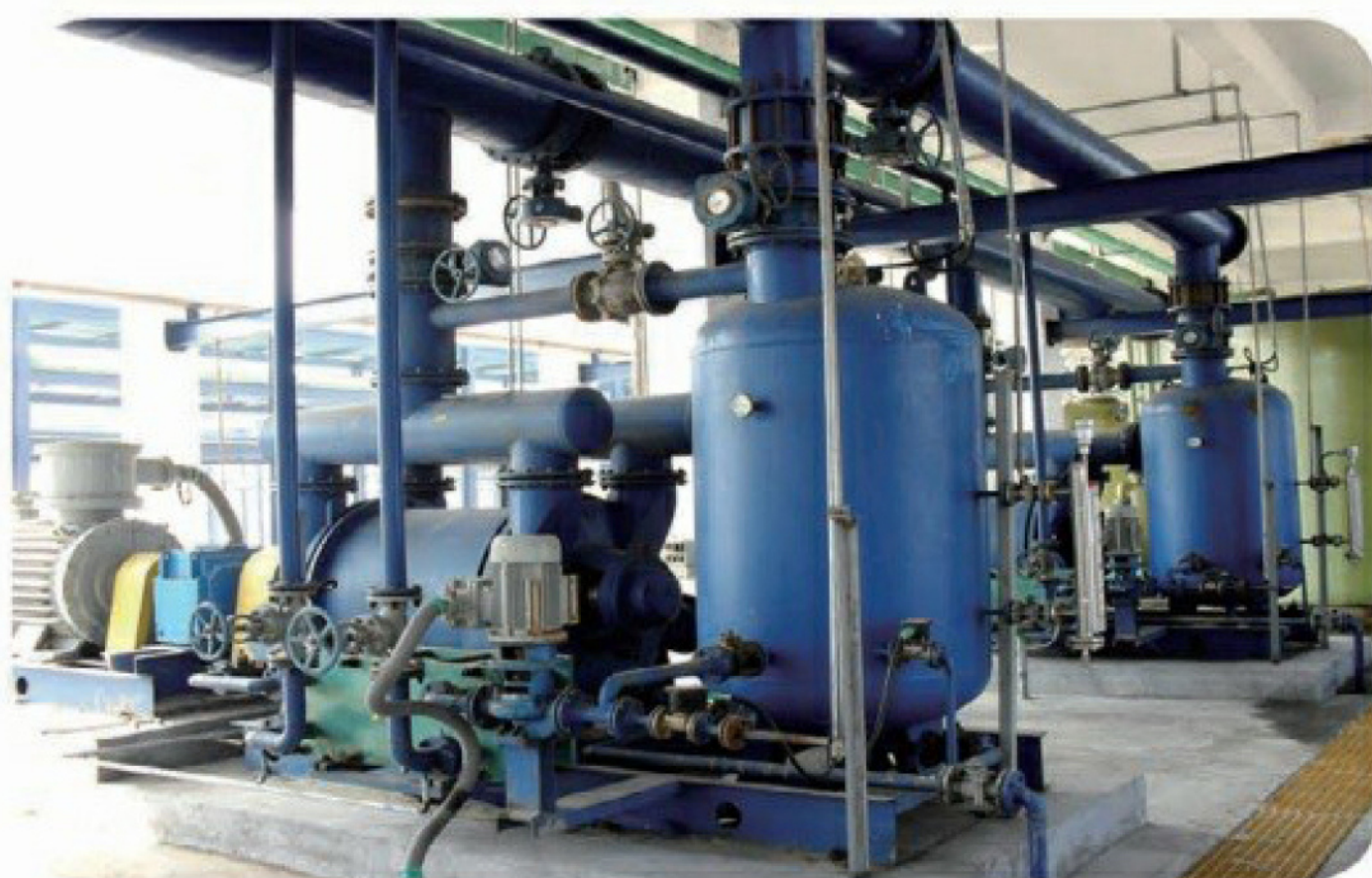
氢气乙炔压缩 Hydrogen and acetylene compression
