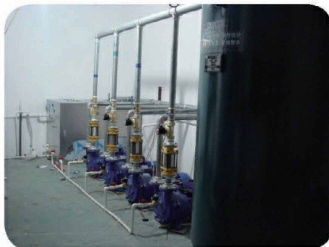
医疗负压站 Medical negative pressure station
